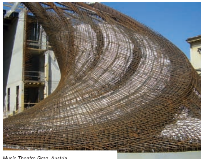
Music Theatre Graz, Austria Engineering Office convex ZT GmbH, Graz
